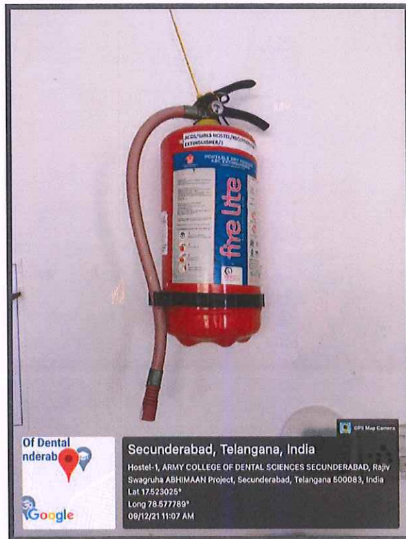
Fig-21: Fire safety equipment in Boy's hostel
