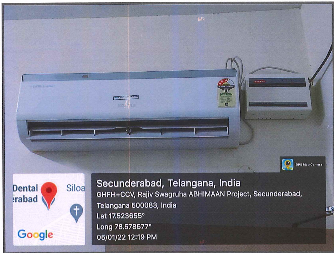
Fig-20: 3-star Air conditioner unit installed in various departments
