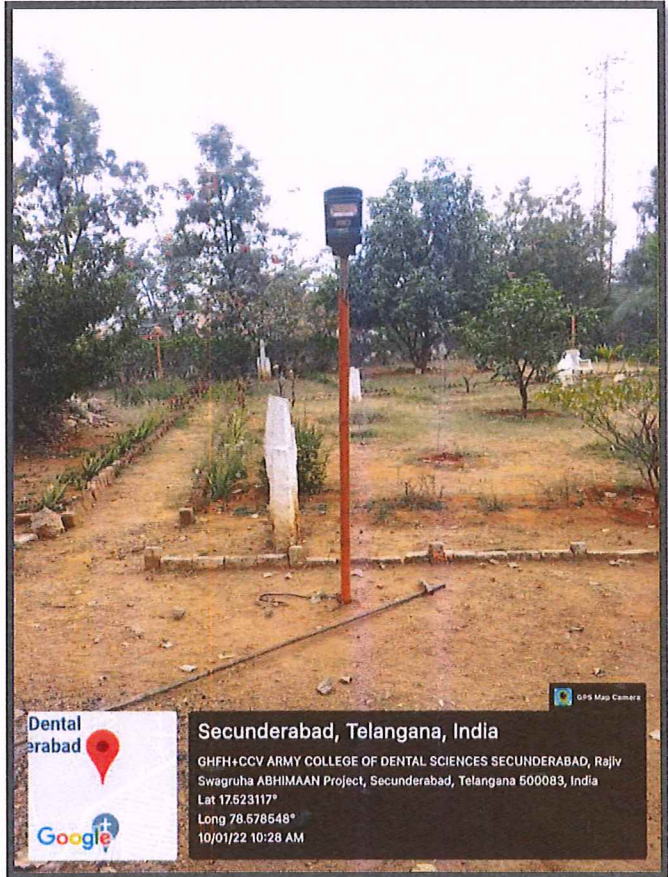
Fig-6: Solar flood light installed in college garden
