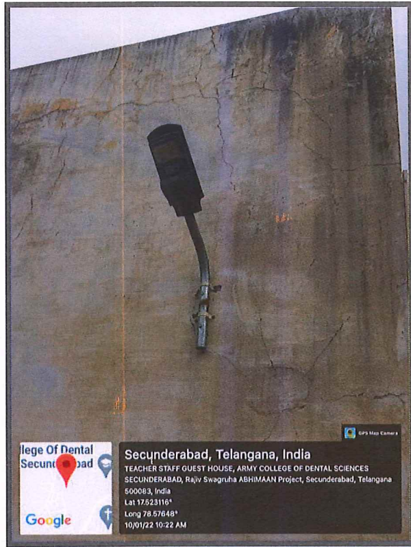
Fig-7: Solar flood light installed near family quarters
