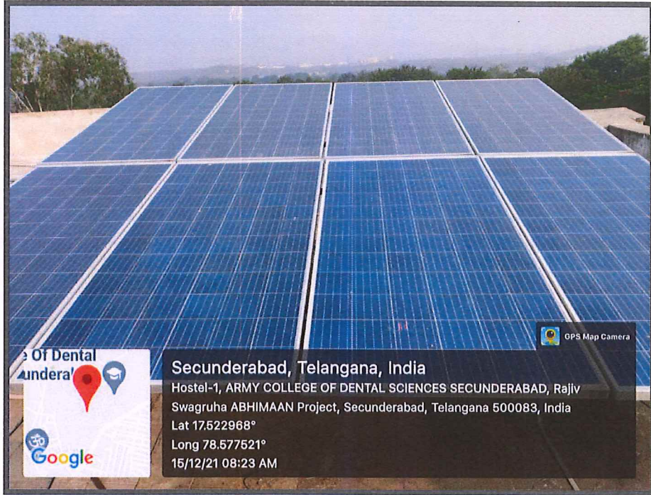
Fig-1: 25 KW solar roof top power grid
